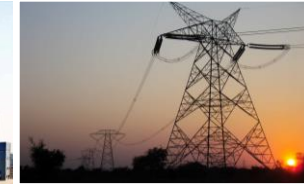
Longest Private HVDC Line in Asia
