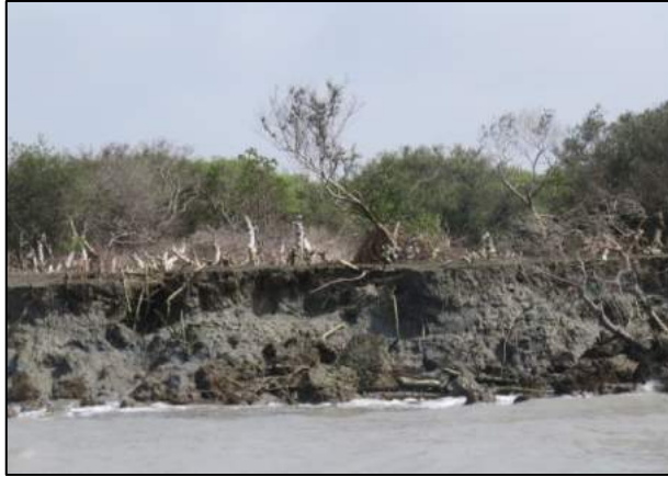
Fig. 15. Erosion of banks of Bocha island along the Navinal creek
