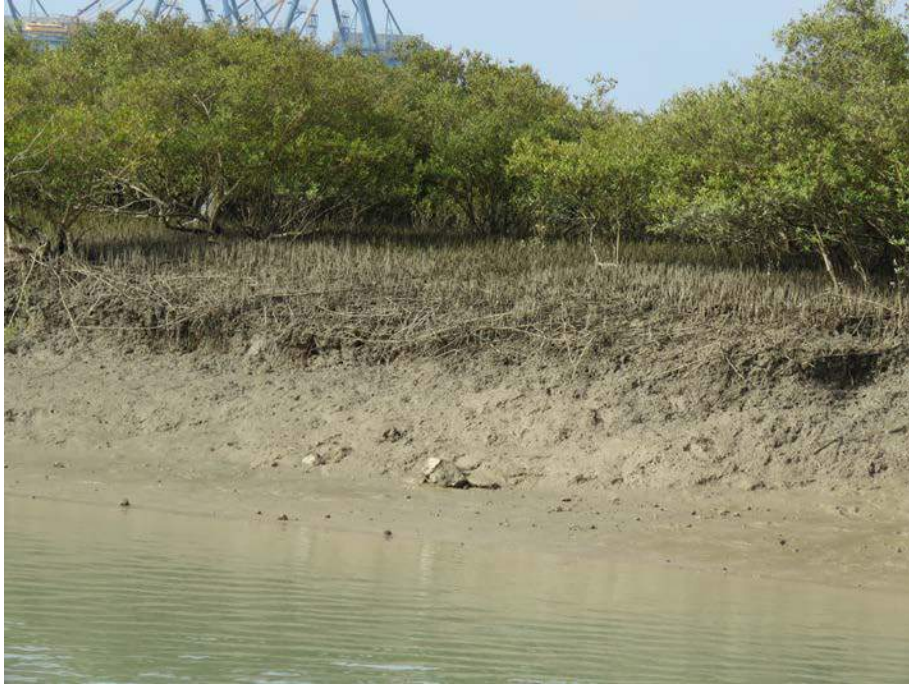
Fig.16. Erosion of banks of Bocha island along Navinal creek
