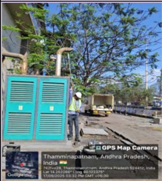
DG SET – SOUTH SIDE 1
