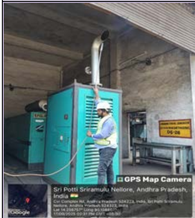
DG SET – ADMIN AREA
