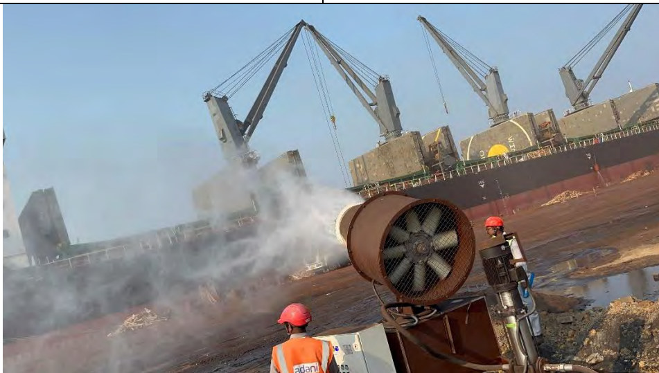
Dust suppression system at south side of the Port
