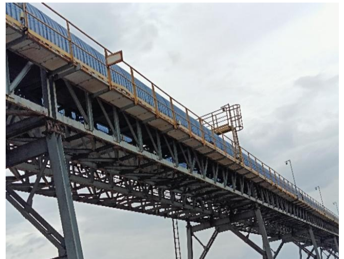
Closed conveyor system for coal Handling
