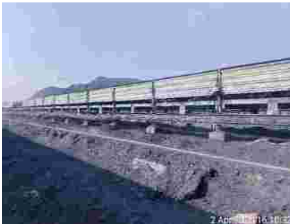
Cladding to conveyor belt
