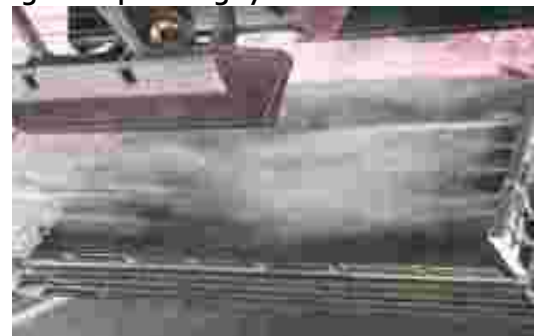
Transfer towers and Vessel loading area sprinkling systems
