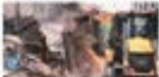
Demolition drive at ITO area in New Delhi, India, following a court order.
