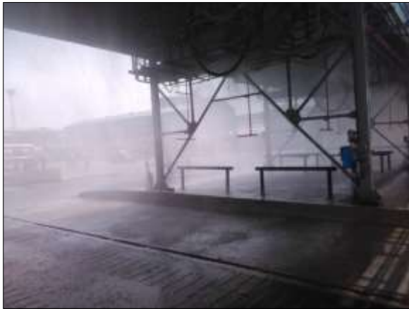
Water sprayed through sprinkler system
