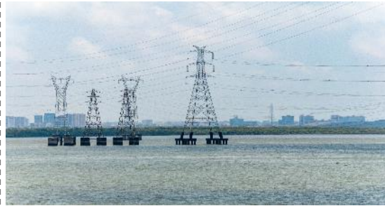
AESL (Mumbai – Vikhroli Transmission Line)
